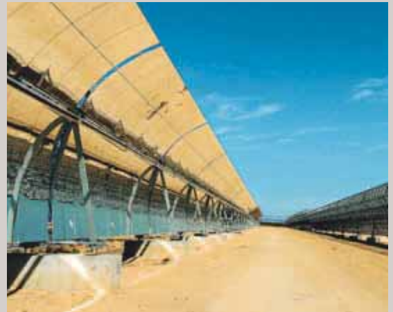
Range of parabolic mirrors © Abengoa Solar.
