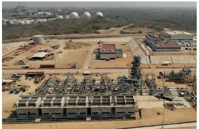
Altamira's re-gasification terminal
