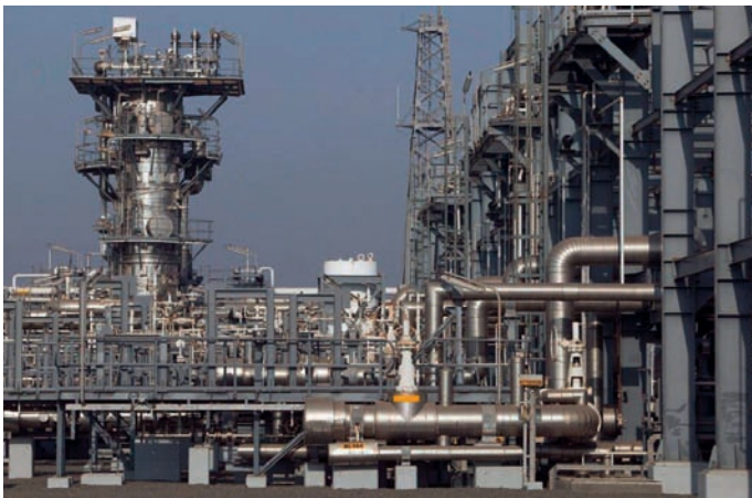
LNG Hazira's re-gasification terminal
