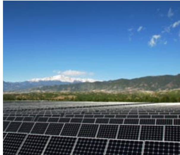
SUNPOWER® OASIS™ C1 POWER PLANT
