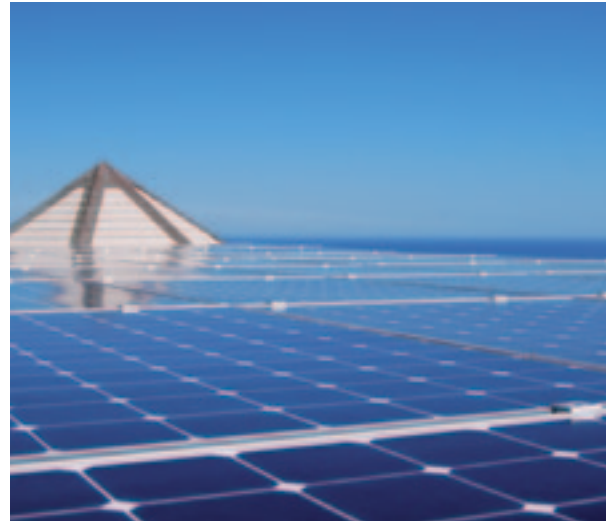
ROOFTOP SYSTEM POWERING RESIDENCE IN CLIFTON, CAPE TOWN.
